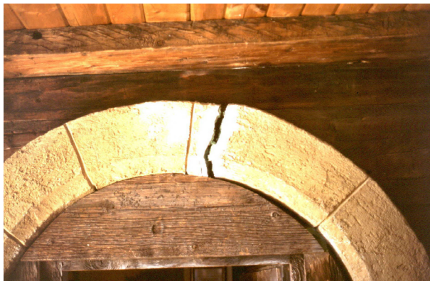
Risse in Türboge, Restaurant Steinegg
